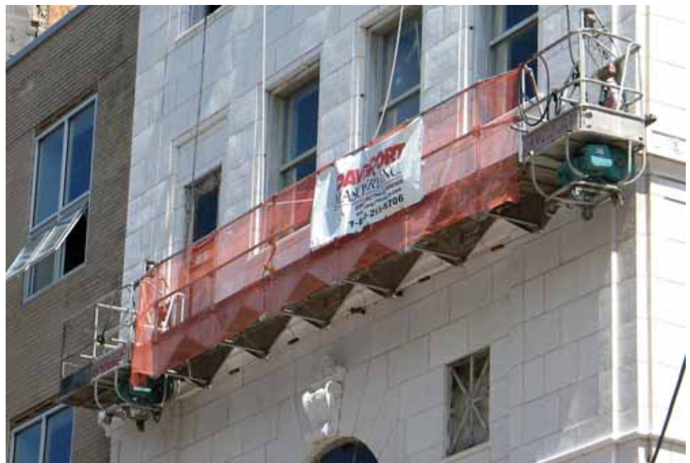
DMI continues to work at the First Street Lofts in Flint, MI
